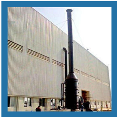
PP Gas Chimney
