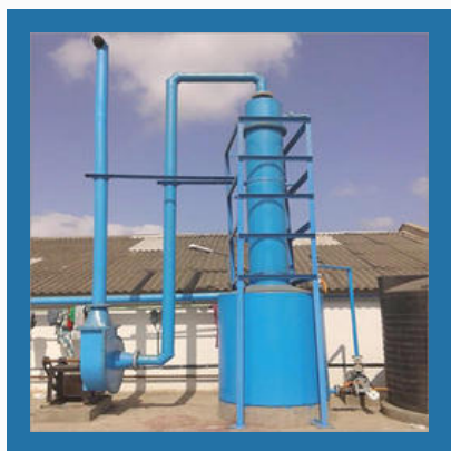
PP Scrubbing System
