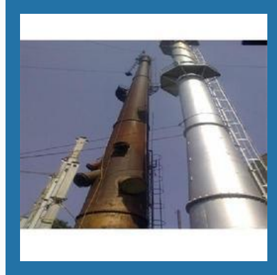
Industrial Gas Chimney
